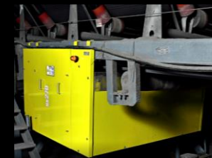
Hx270-1 TOP COVER MONITORING DEVICE
